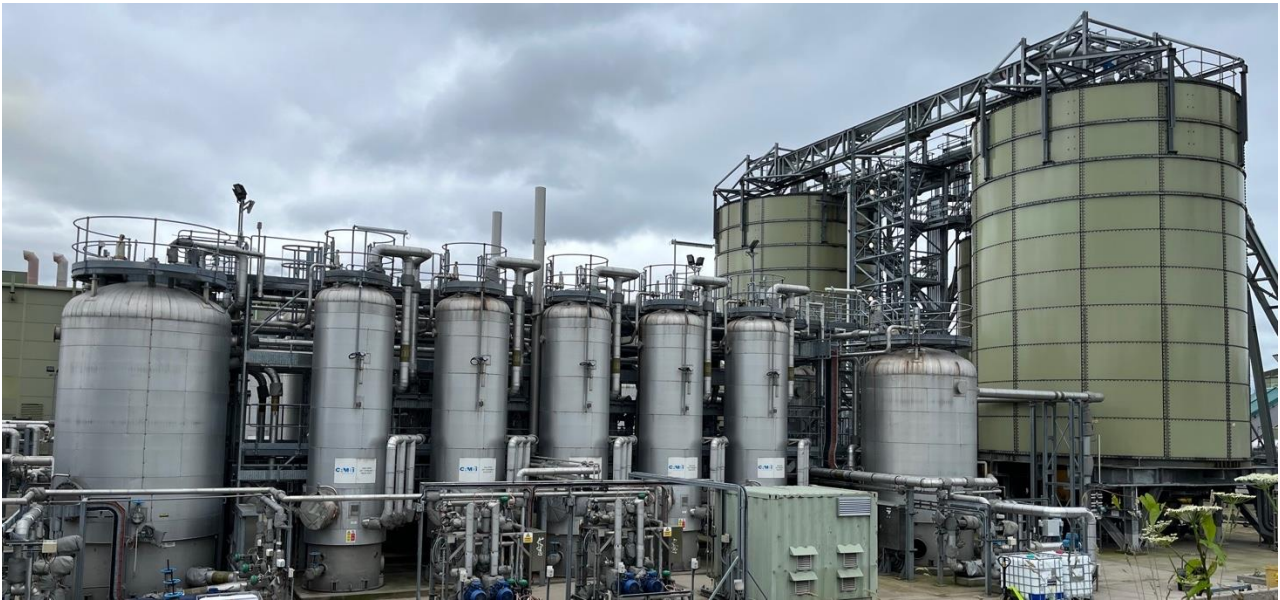
Figure 5-9: Davyhulme WWTW sludge storage soils (right) and Cambi process tanks (centre), UK, June 2024
