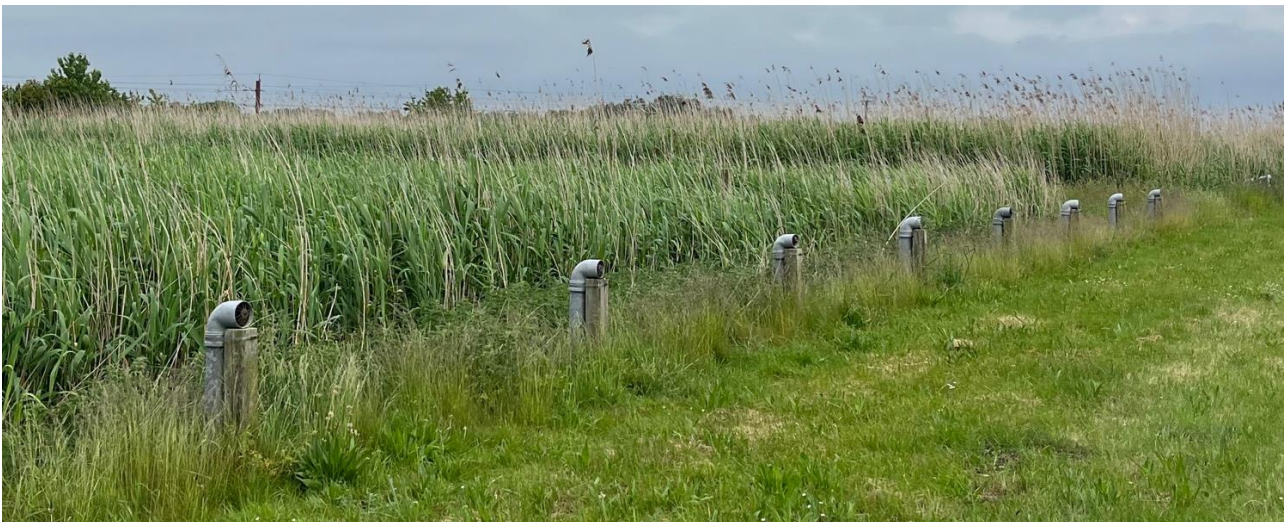
Figure 5-7: Air ventilation pipes (which become the filtrate pipes), Greve STRB, Denmark, May 2024
