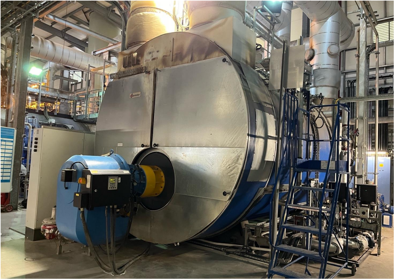
Figure 5-11: One of Davyhulme’s biogas-powered boiler units which provides steam to heat the Cambi process tanks, UK, June 2024
