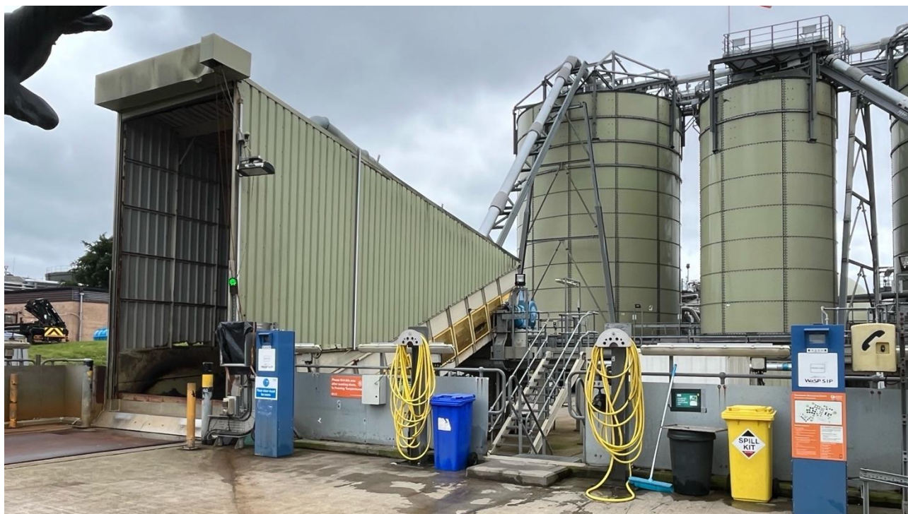
Figure 5-8: Davyhulme WWTW sludge receipt area, including truck washing area, weighbridge and storage silos, UK, June 2024
