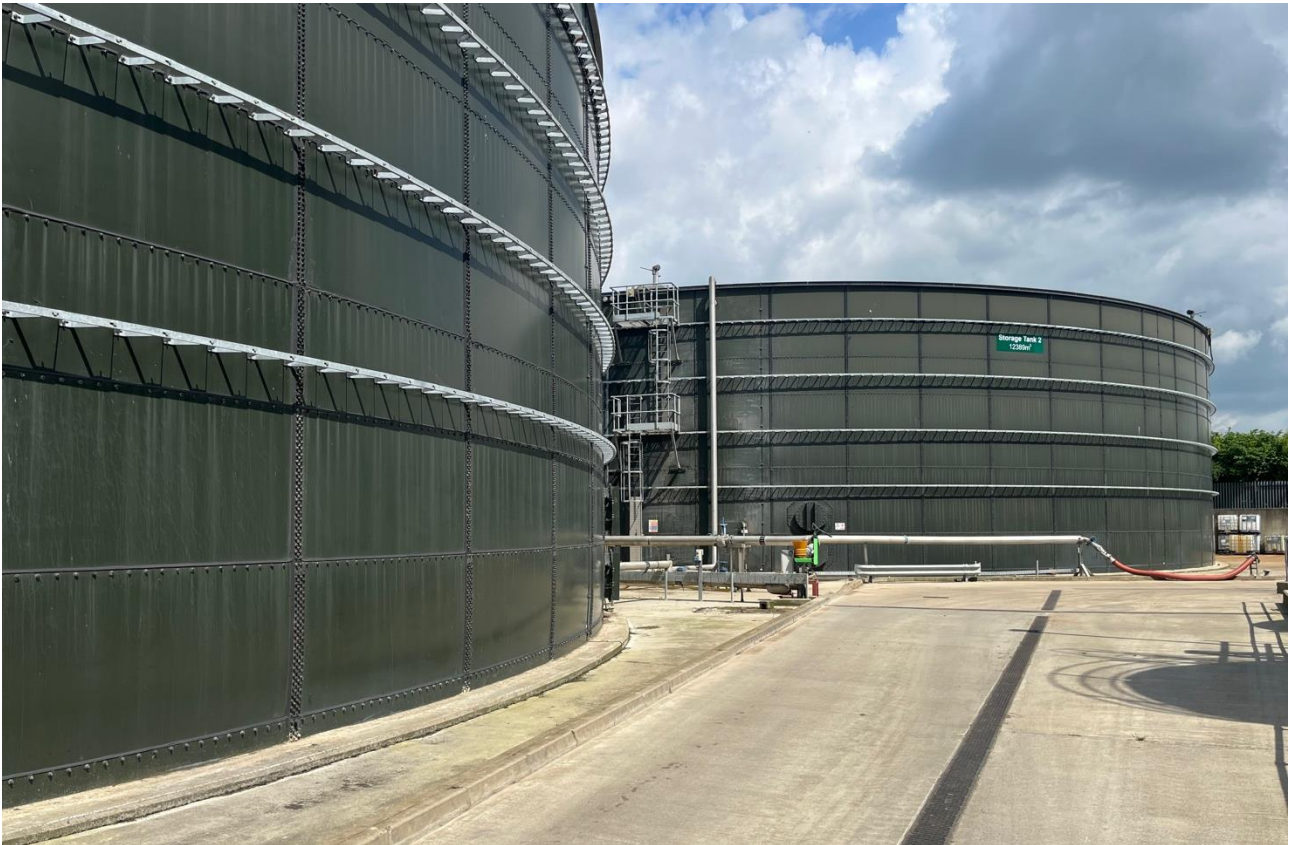
Figure 5-4: Biogen Bygrave digestate storage tanks, which store digestate outside of the land application season, UK, June 2024
