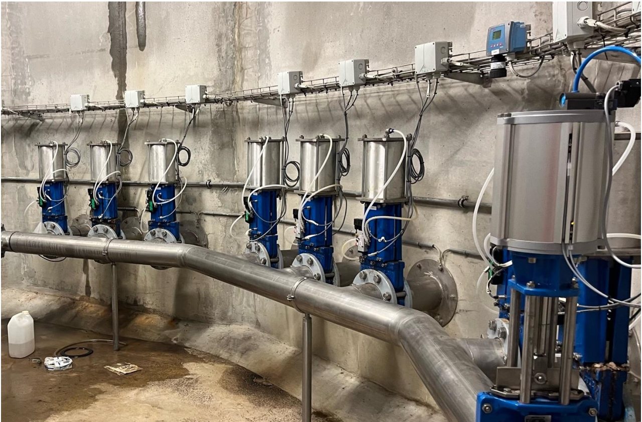
Figure 5-6: Valves on the sludge loading (influent) pipelines, located in a dry well adjacent to the reed beds, Haslev STRB, Denmark, May 2024
