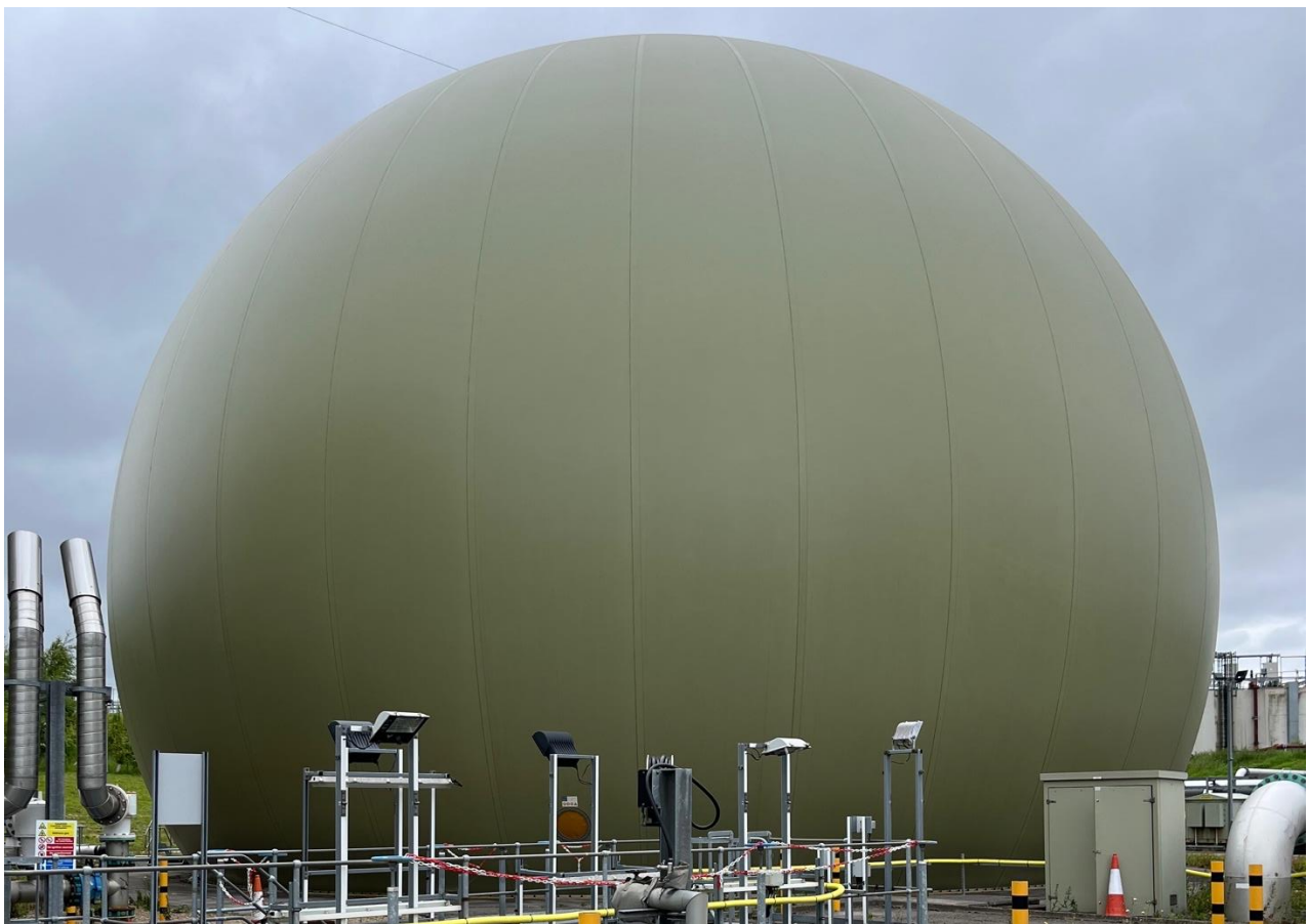
Figure 5-10: One of two 9,000 m 3 biogas storage tanks at the Davyhulme WWTW, UK, June 2024
