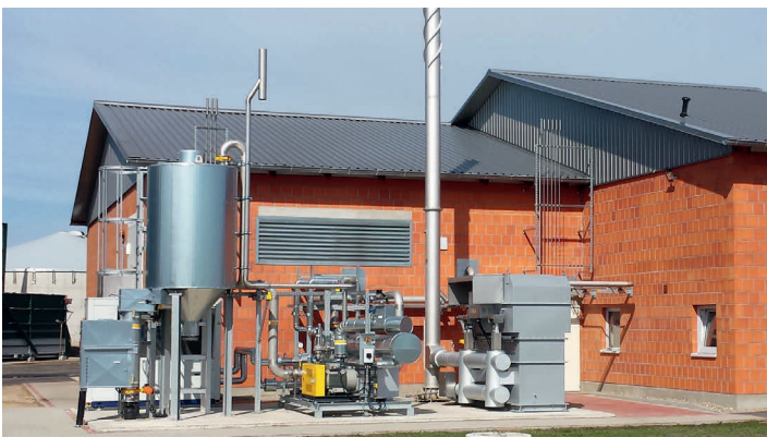
Outdoor installation of raw biogas pre-conditioning and exhaust gas treatment
