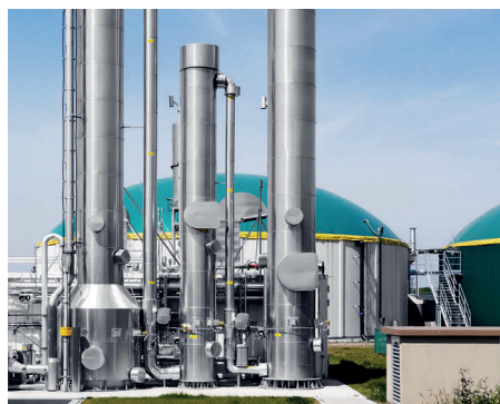
Biomethane plant Semd - Germany
