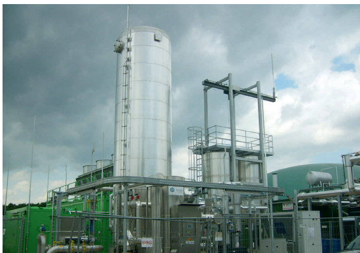
Biogas treatment plant Neudorf (Brandenburg-Germany), 700 Nm 3 per h BioMethan, amine wash process
