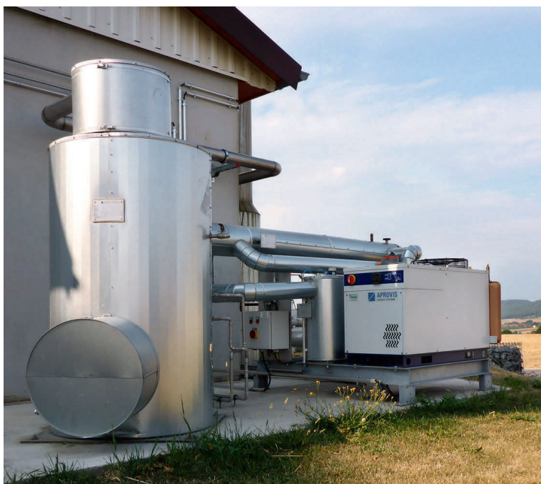
External insulated desulphurisation-unit (activated carbon) and cooling unit for dewatering
