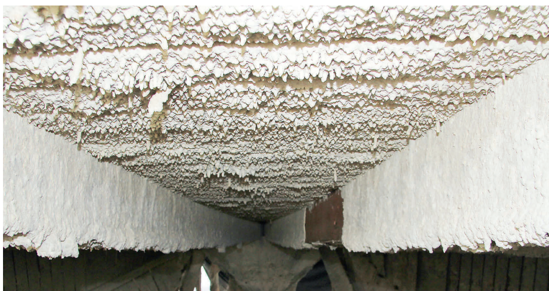
Elementary sulphur accumulates e.g. at the roof of the digester
