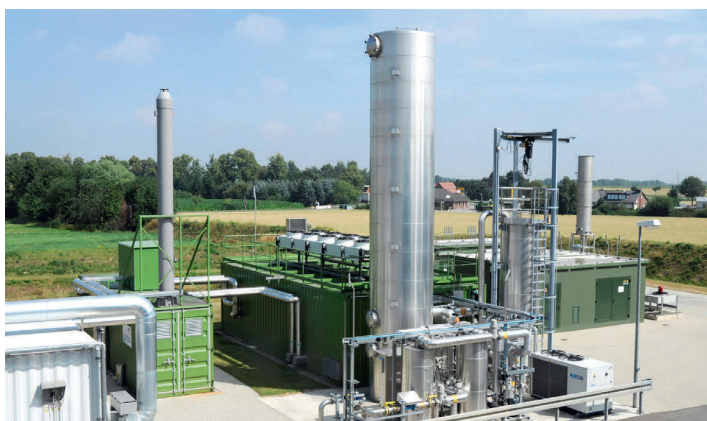
Heat-led gas upgrading process – Plant for biomethane production with pressureless amine scrubbing in Bruchhausen-Vilsen
