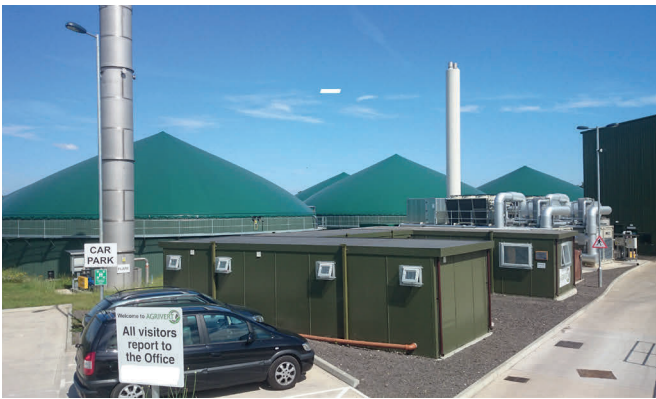
West London facility with bwe anaerobic digestion technology has been awarded two times in a succession as the best merchant waste AD project
