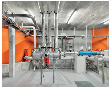
Pump room of the biogas plant Recycling Energie AG
