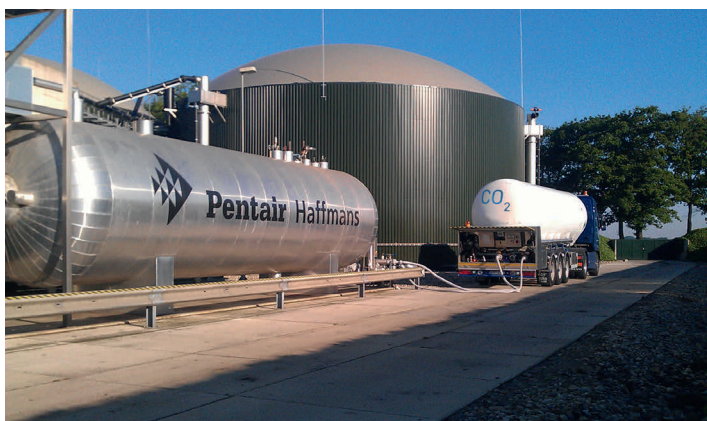
Biogas plant and CO 2 buffer tank
