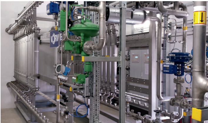
Indoor installation of membranes for CO 2 separation
