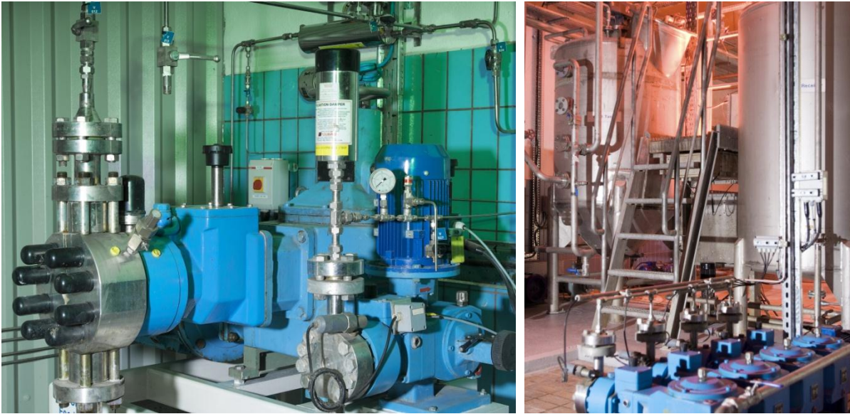
Figure 9. Photos of supercritical wet air oxidation plant treating sludge. [Courtesy Scfi]
