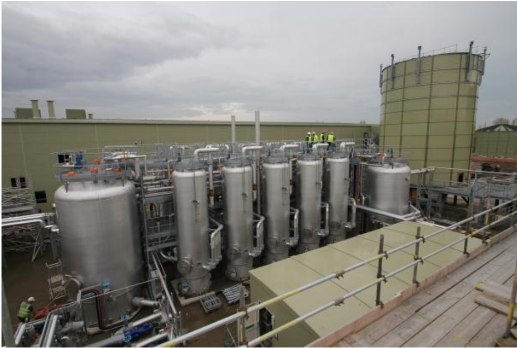
Figure 7. Early installation photograph of Cambi thermal hydrolysis plant being installed in Davyhulme, Manchester. It will have a processing capacity of 121,000 tonnes dry sludge per year. [Photo: Cambi]
